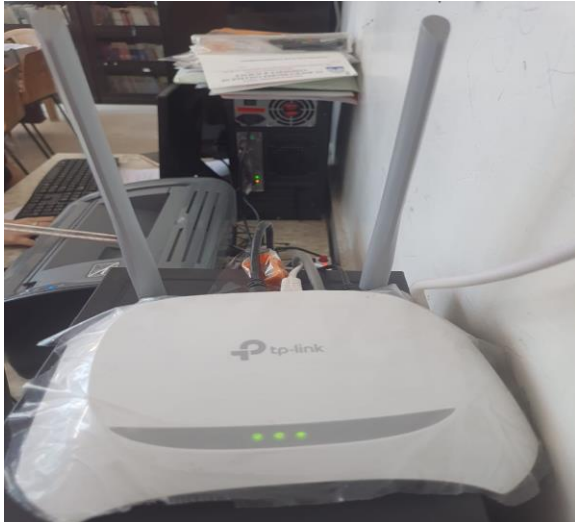
WIFI ROUTER FACILITY
